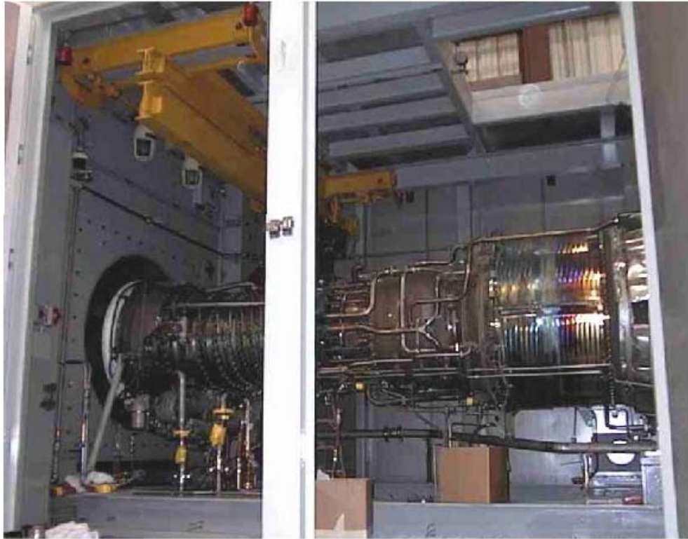
Figure 8 Gas turbine module within housing
