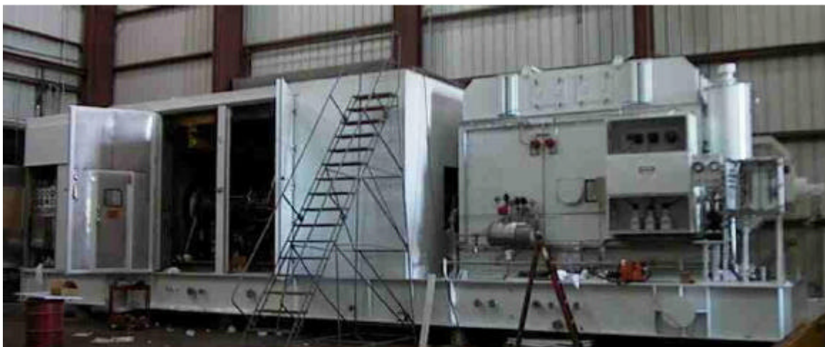
Figure 10 Gas turbine and generator assembly
