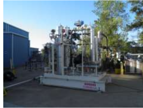
Gas mixing skid
