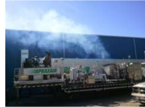
CO 2 tank and vaporizer
