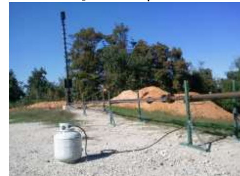
Gas flare system
