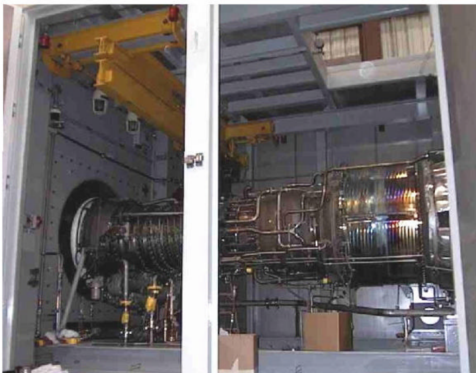
Figure 8 Gas turbine module within housing
